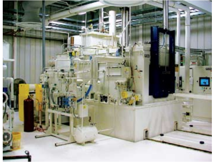
NHBB's vacuum carburizing furnace.
